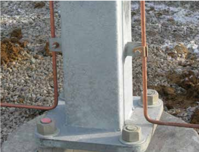
Substation earthing riser
